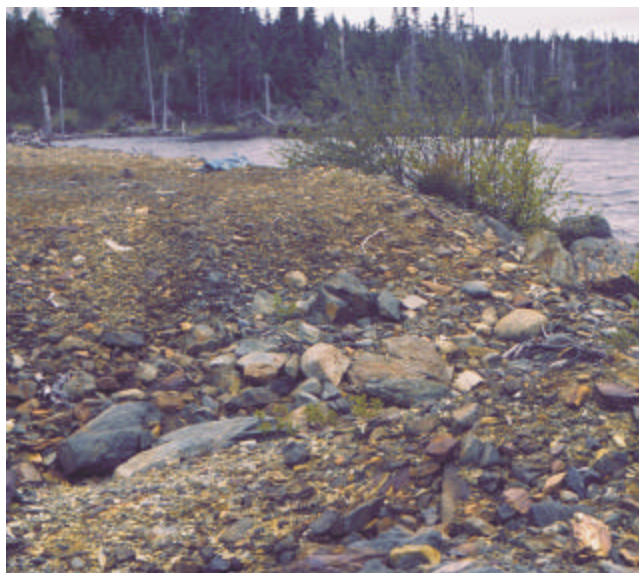
Plate 1. Looking southwest from tailings pond across breach in dyke into Little Rambler Pond. Note the abundance of weathering, sulphide-rich, waste rock used in dyke construction.
